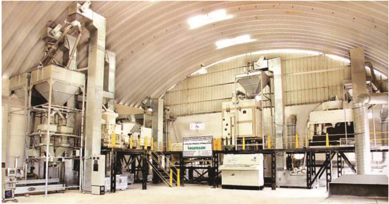
Seed Processing Plant: Capacity 8 TPH with Central Dust Aspiration System. Installed on raised platform
